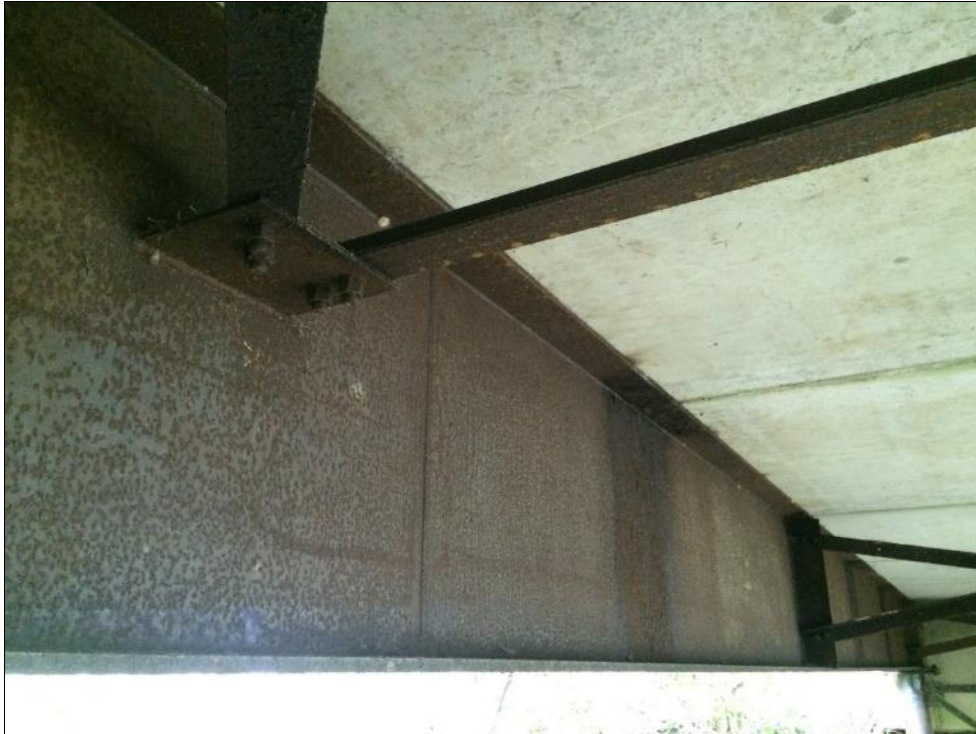
Photo #17 Interior face of girder /underside of deck
